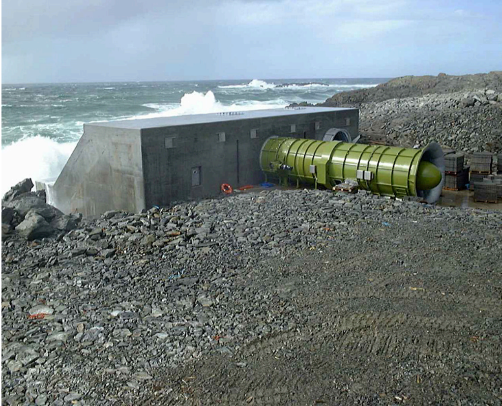
Figure 9: A photo of the LIMPET wave energy turbine system installed in Scotland
